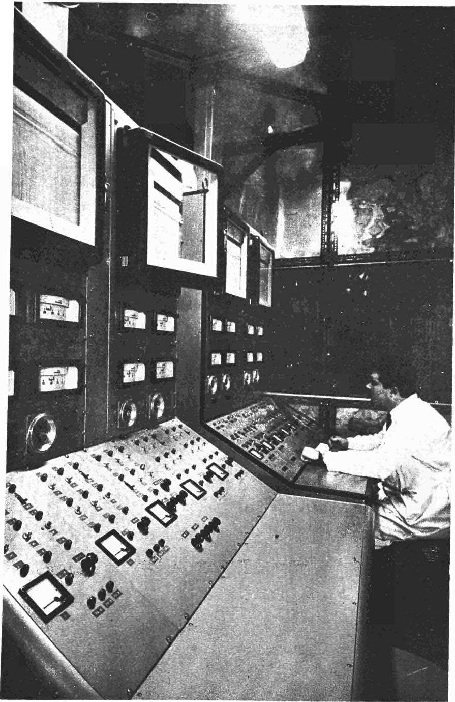
Fig. 4 : View of the control room and control desks
