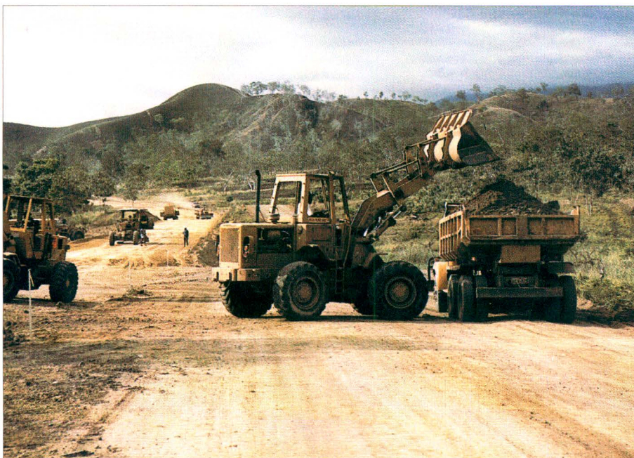
Much of EU-PNG cooperation has focused on improving the country's inland road network
