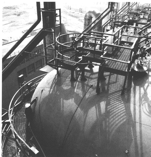
An example of acoustic monitoring of corrosion cracking in Cowper stoves, showing acoustic emission transducers attached to the stove dome.
