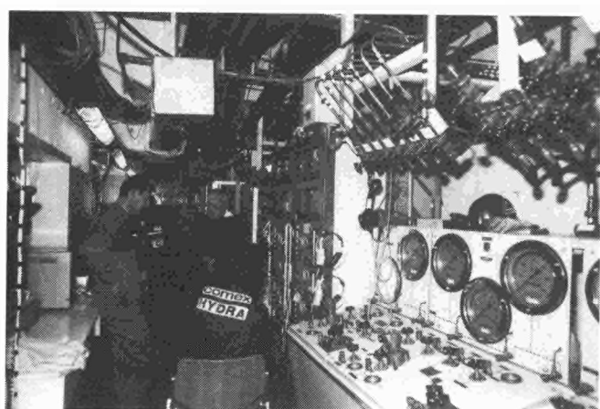
Decompression control room aboard DSV 'Orelia'
