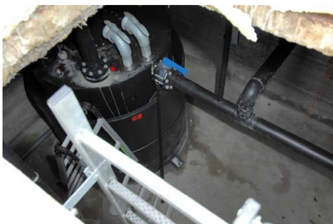
Waste water tank
