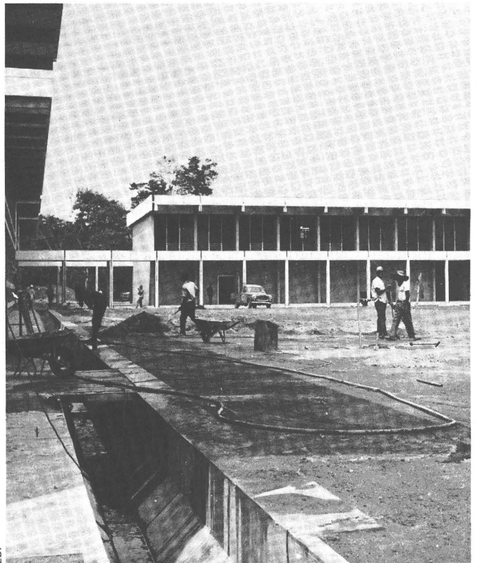
"The EDF has concentrated on buildings rather than on technical assistance". A college of education in Brazzaville (Congo) the construction of which was financed by the EDF
