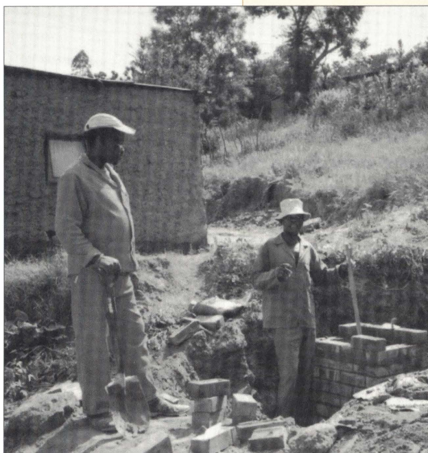
Desai residents install a tap - gaining essential services and valuable skills for the jobs market.
